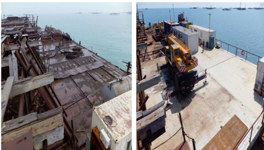
BH Platform 83/162 Production Deck – photographs of before and after 2016 refurbishment. Source: Company
